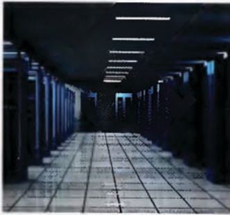
5 Digital switching equipment
